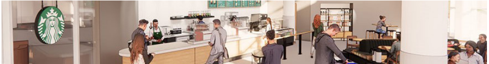
Construction for the Starbucks Café project in the Student Engagement Center took place over the summer in time for a grand opening, Aug. 22, on the first day of classes on the Broadway Campus. Sodexo expects to hire at least 20 students for part-time jobs.
